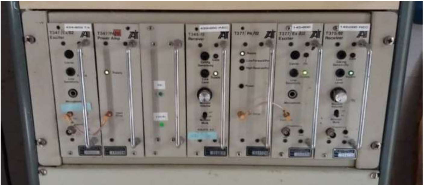
70cm and 2m transmitters and receivers inside the equipment building. Third module in from the left is the site microprocessor controller.
