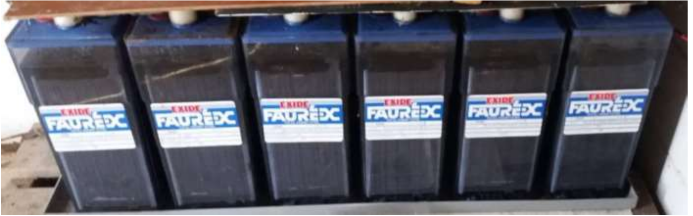
The site has mains power and for back-up a bank of six 2V lead acid batteries keep the site fully operational during occasional power out-ages.
